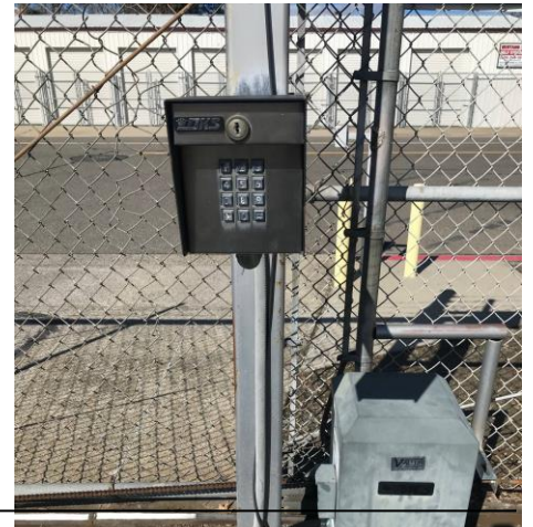
Controlled Access Security Gate Access Panel Box for entering PD along D St.
